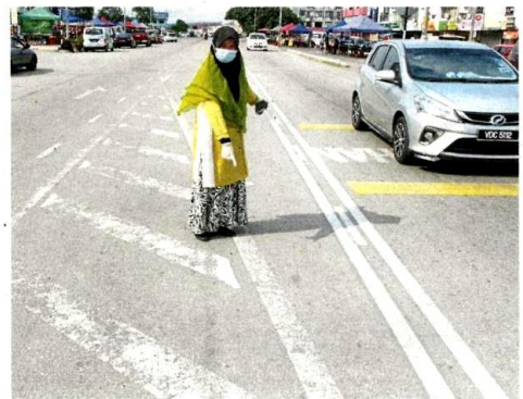
Dr Halimah says motorists may end up in the opposite lane at night because they cannot see the faded road lines. — KK SHAM/The Star
