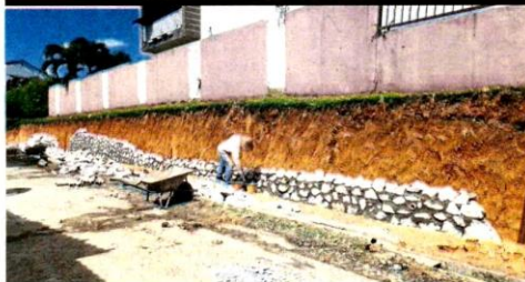
SMK Assunta's retaining wall has been repaired, thanks to an allocation provided by the state government for partially aided schools.
